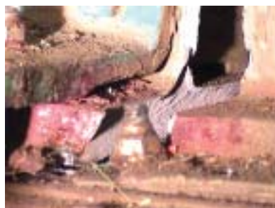
A close up of the crack initiation site
