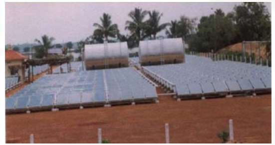
1.2 lakh litre per day system at M/s Godavari Fertilizers, Kakinada
